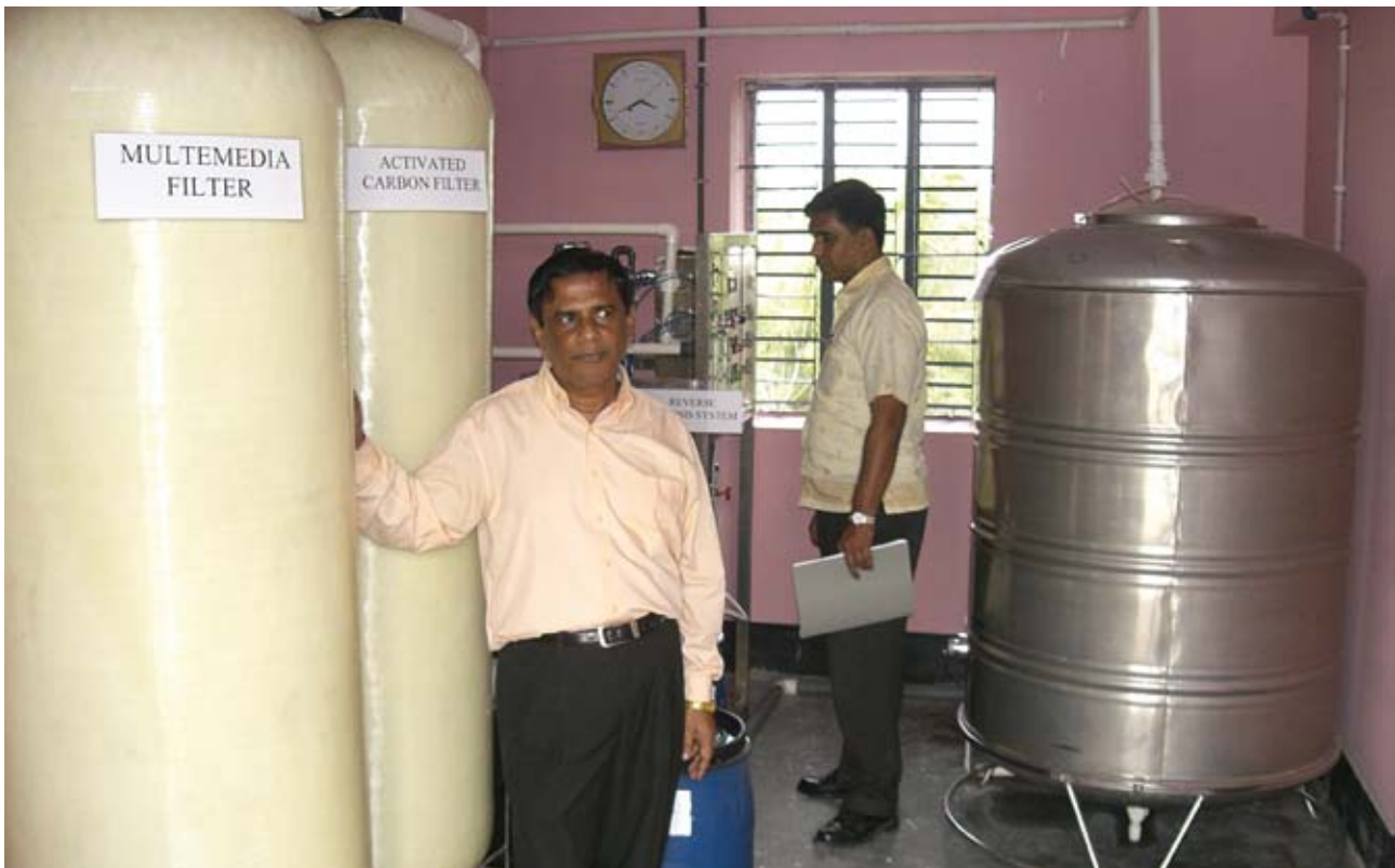
Shelter and safe drinking water is often the most pressing need, when a cyclone hits the community. Photo: Brot für die Welt
